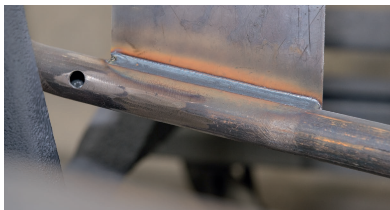
Thin steel plates with thicknesses between 1.0 and 1.6 millimetres are welded to the base frame. The Lorch SpeedCold welding process only applies the energy currently required.
